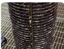
Before Treatment Heavy Struvite Build-up
